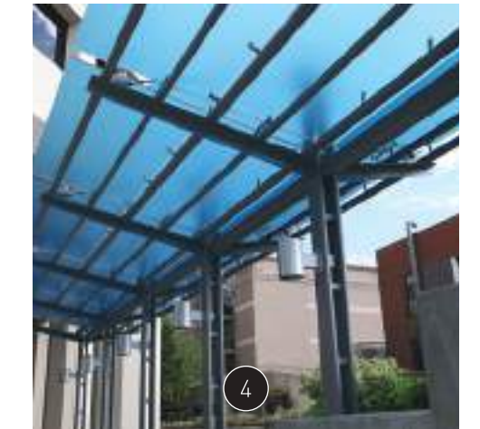
4 MADE IN THE SHADE A sun shade structure makes a cool statement and provides a safe haven from the elements.
